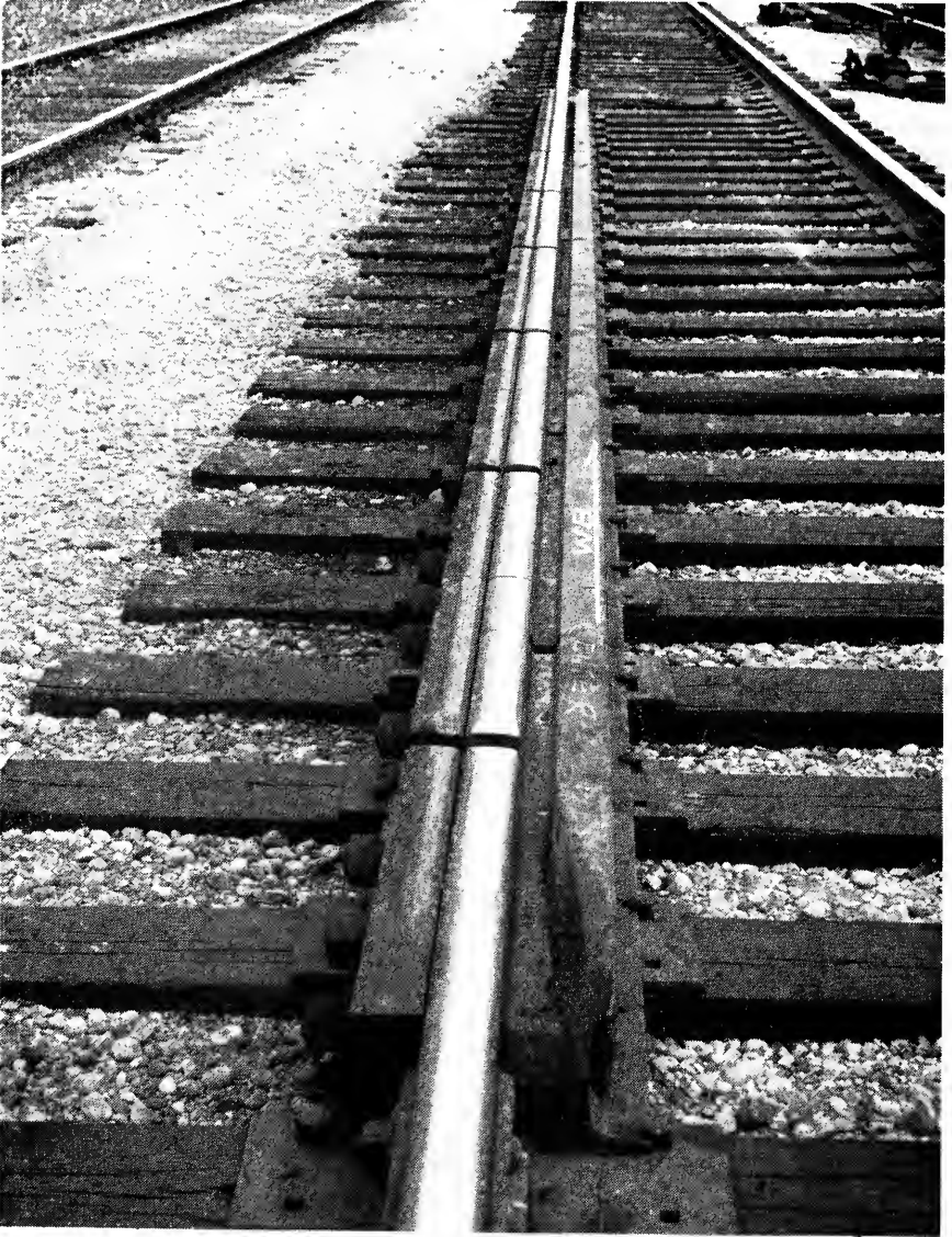
Fig. 2. View of Center Test Panel After 3 1/2 Months' Traffic (The first flangeway in the foreground is in the unit with unhardened control cooled rail).
